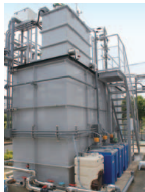
Wastewater processing system
