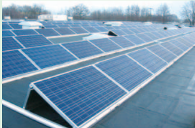
Photovoltaic system installed at the Neumünster Factory
