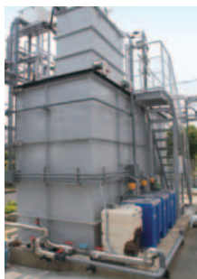
Wastewater processing system
