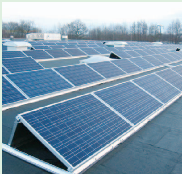
Photovoltaic system installed at the Neumünster Factory
