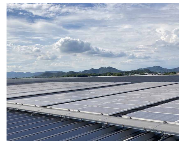
Solar panels (i-Square)
