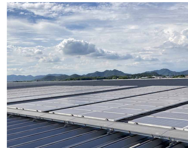
Solar panels (i-Square)
