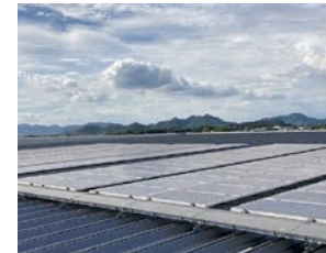
Solar panels (i-Square)
